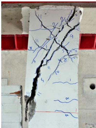
側位移比1.5%，斜向裂縫貫穿短柱
