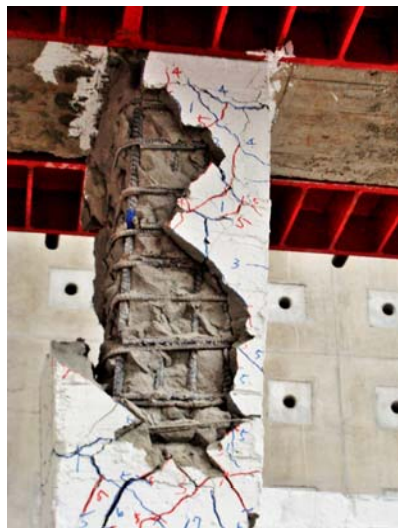
側位移比1.75%，混凝土嚴重崩落
